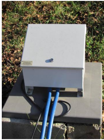
In order to remove iron from the discharge, an aerator is used and run by this generator which is powered by renewable energy on site.
