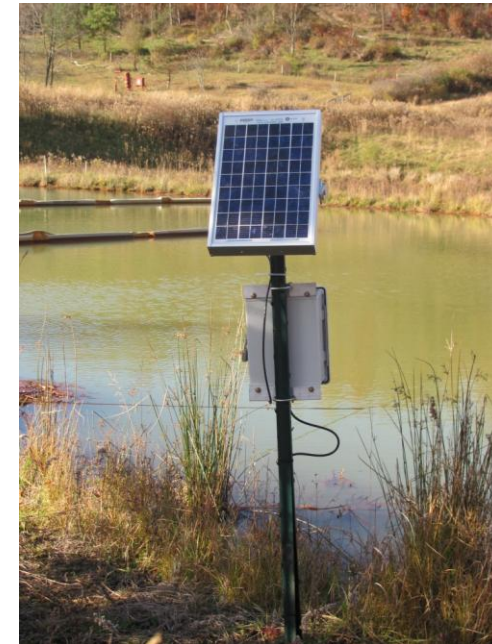
This panel powers a probe that monitors water quality 24/7
